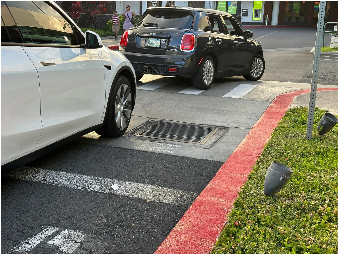
As you can see the concrete surround on this storm drain is so damaged that the rebar on the left side in this photograph is exposed. This is near the crosswalk and in an area where folks, disabled and otherwise, frequently walk.
