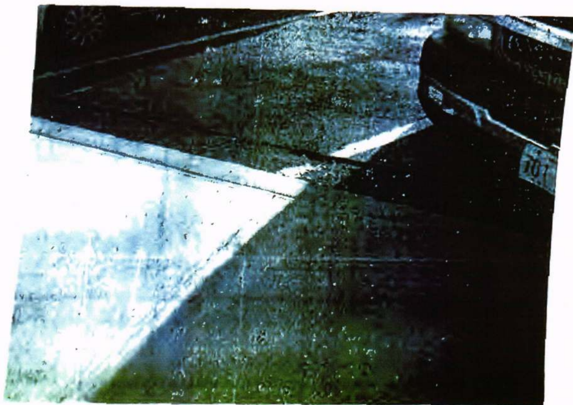
Figure 2: Close-up View of Area Where Ms. Romano Stepped Down onto the Parking Lot Surface
